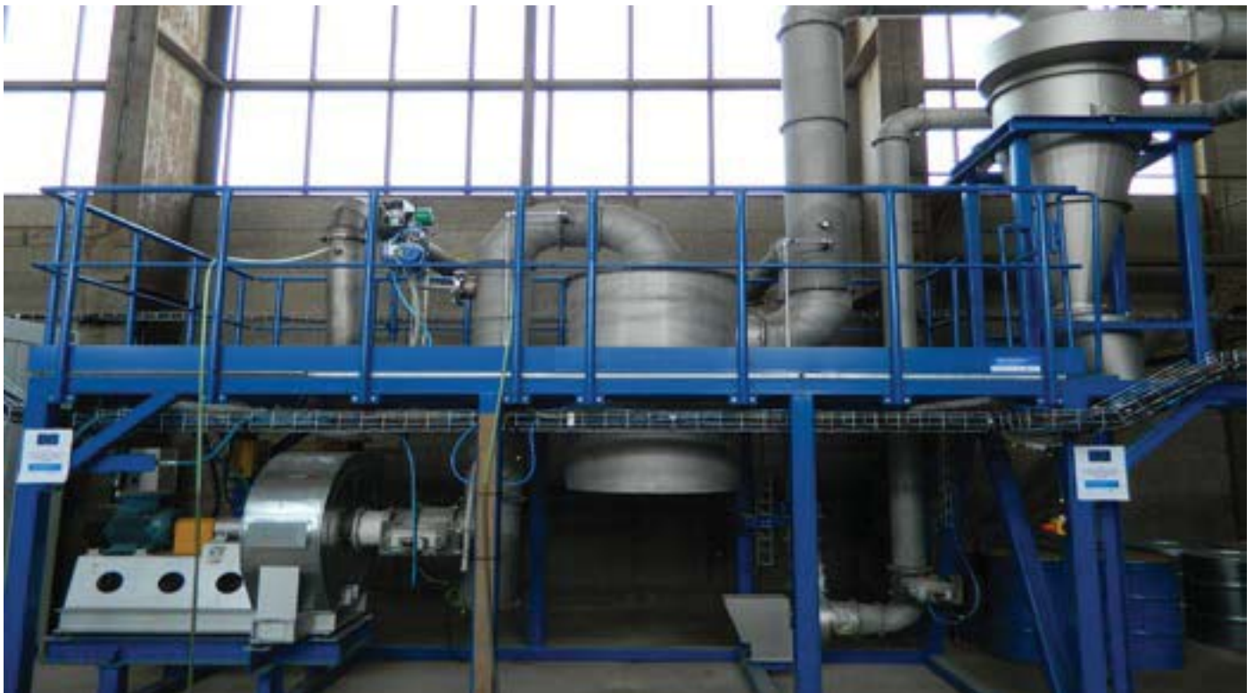
Fig. 2 Off-gas pre-treatment module of continuous thermal desorption pilot unit.
