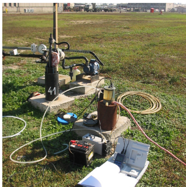
Monitoring well with continuous monitoring of process parameters
