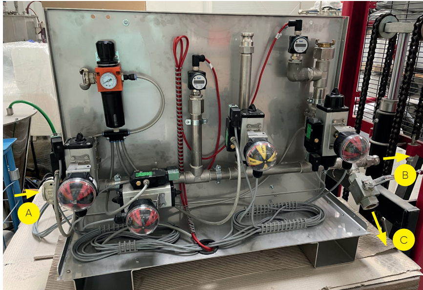
A - Inlet of suspension from the pump B - Outlet of the suspension into the injected well C - Depressurisation valve
