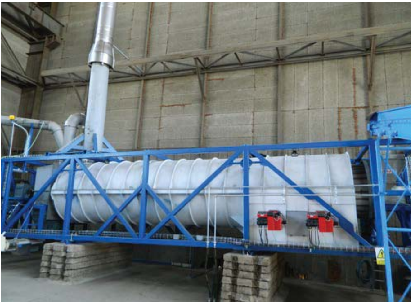
Fig. 1 Rotary kiln of continuous thermal desorption pilot unit.
