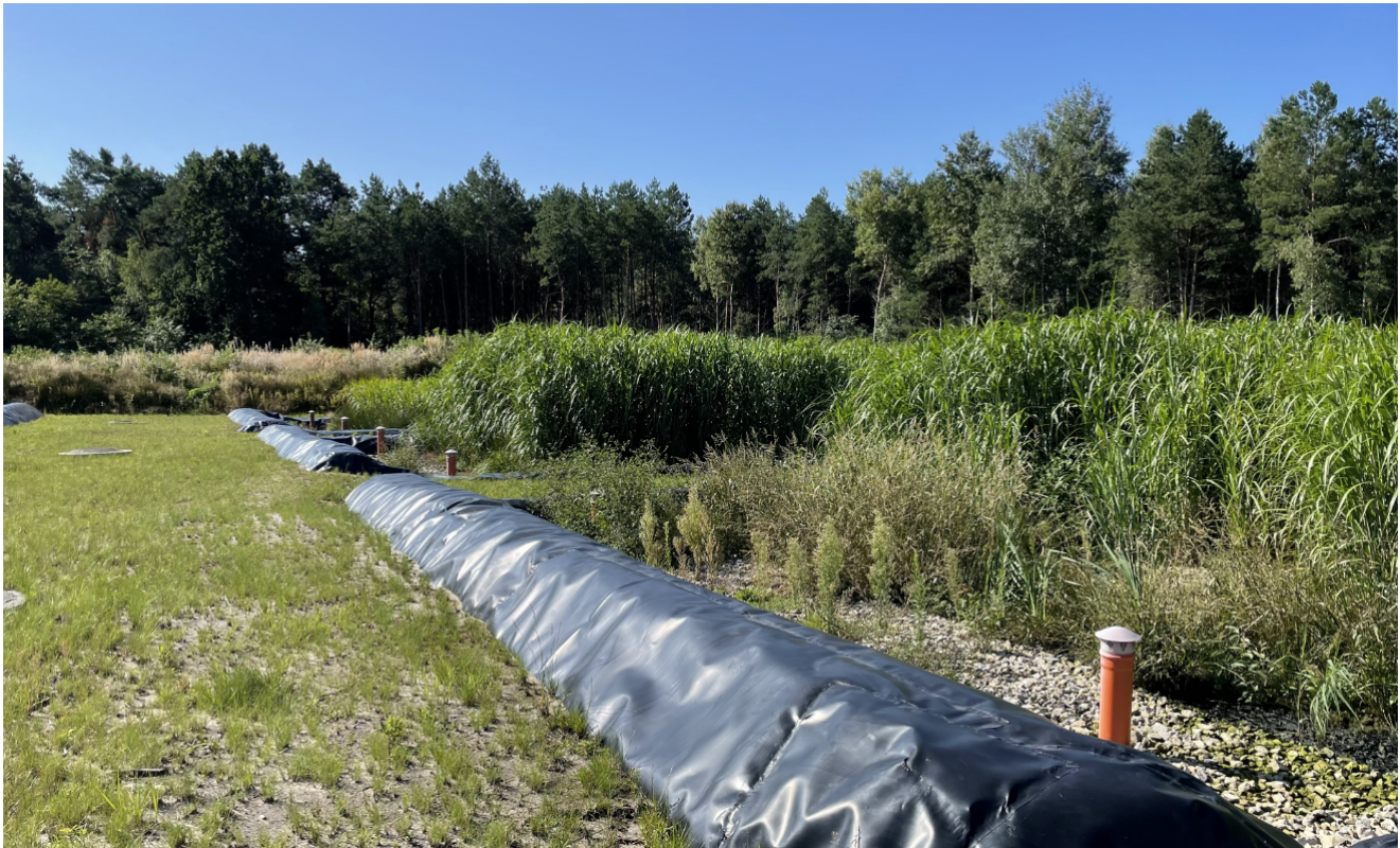
Root wastewater treatment plant in Bialka, Poland (one year after commissioning)
