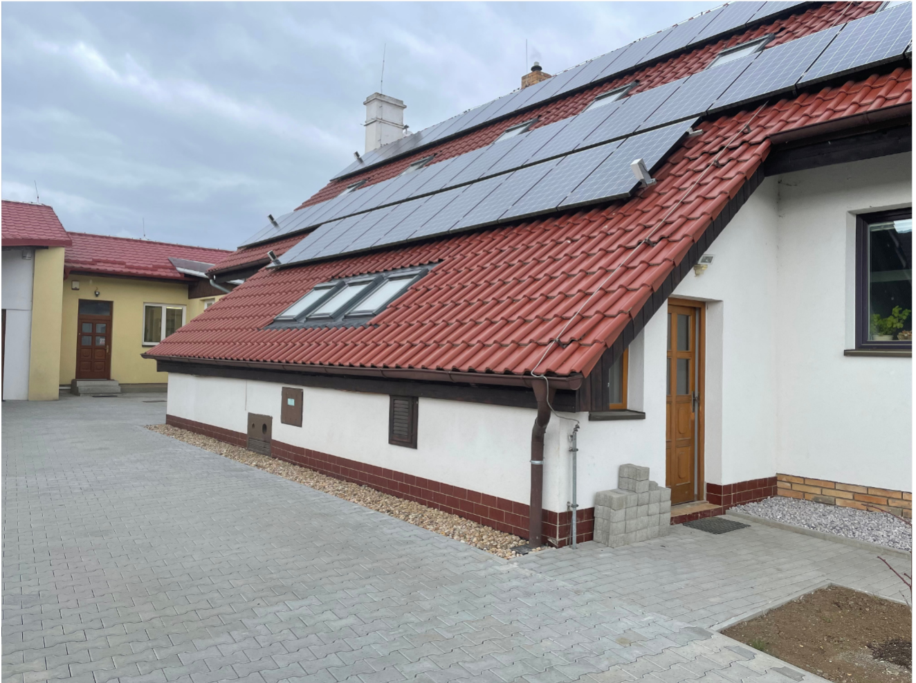
Photovoltaic power plant on the roof of the Dřetovice facility
